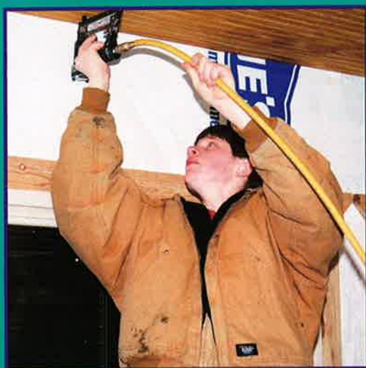
Logan McMurtry staples a roof to the porch of a house for Area 30.
