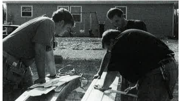
Matt Livesay and Alan Stacy help cut the siding for a house on the job site of Habitat for Humanity.
