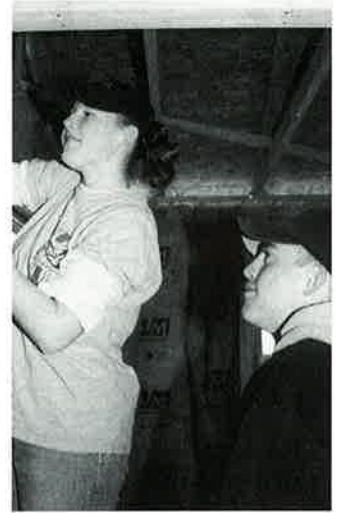
Right: 2000 grad Ben Majors watches as Debra Clarkson uses the staple gun to put up some insulation.
