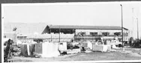
By the end of May, the new middle school structure had begun to take shape.
